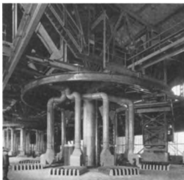
FIG. 5. Charging floor showing top of furnace bins and telfer for charging raw materials.
