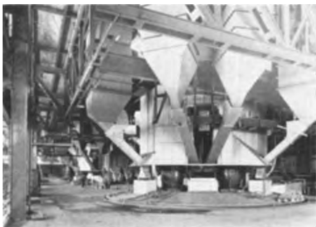
FIG. 4. View from the furnace platform showing three completed 20,000 kw Tysland-Hole furnaces at A/S Norsk Jernverk.
